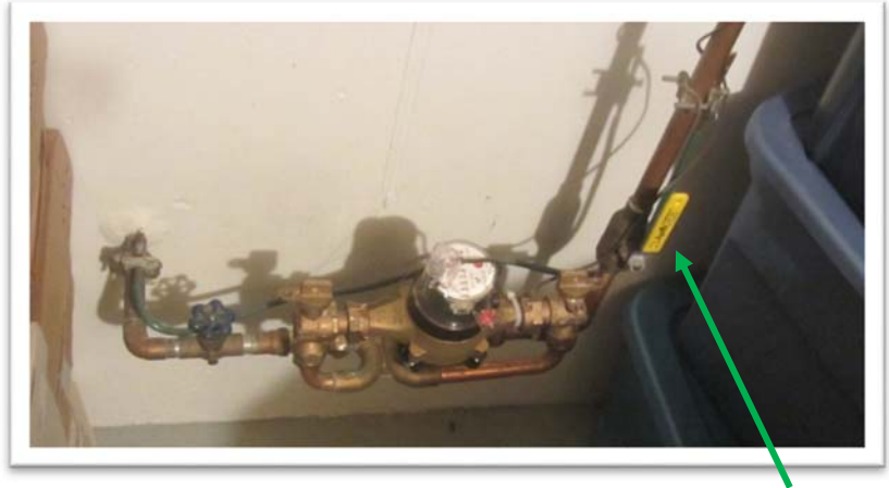
Typical water meter installation with shut-off valve open.
