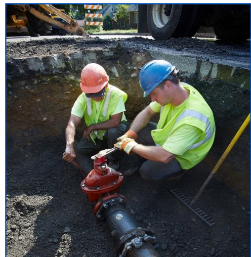
Water Mains 50-100+ Years Old Replace 4+ miles per year - $7M annually
