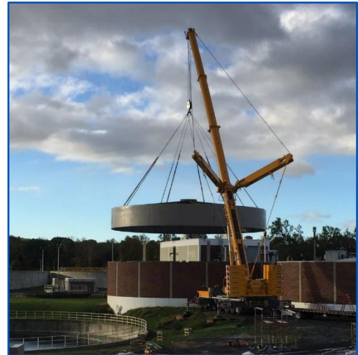
Kline's Island Wastewater Plant Digester Covers Installed 1960s Replaced in 2017 - $3M
